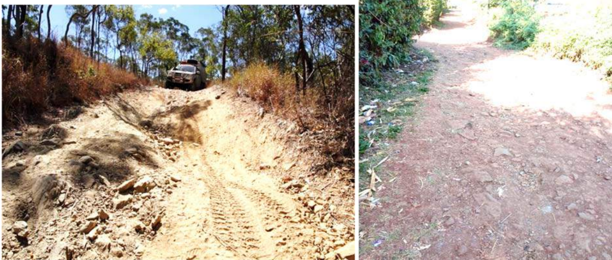
Image 8.1: Rural roads in poor condition, in Matasia
