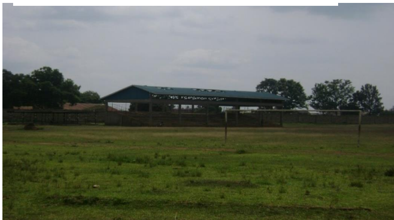
Plate 3-6: Stadium Pavillion with blown-off roof
