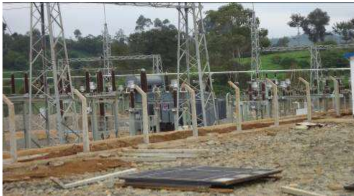
Figure 5: Githambo Power Sub- Station
