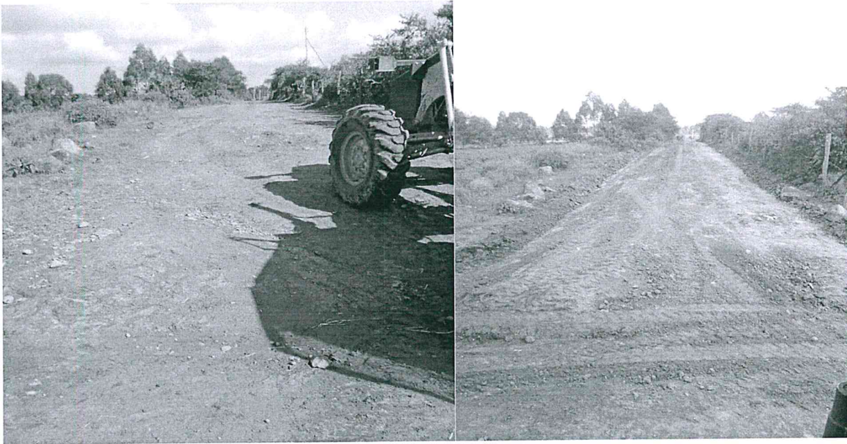
Road improvement under leasing program- Before and After Kahuho Primary Road-Githiga ward
