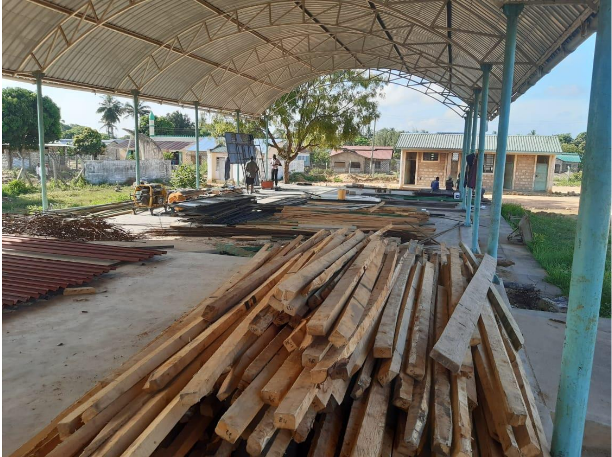
Work is on-going for the construction of the Kombani fresh produce market
