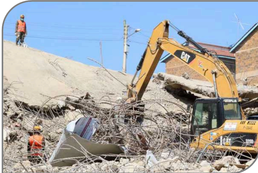
Figure 9:KDF Assisting at a Collapsed Building Site
