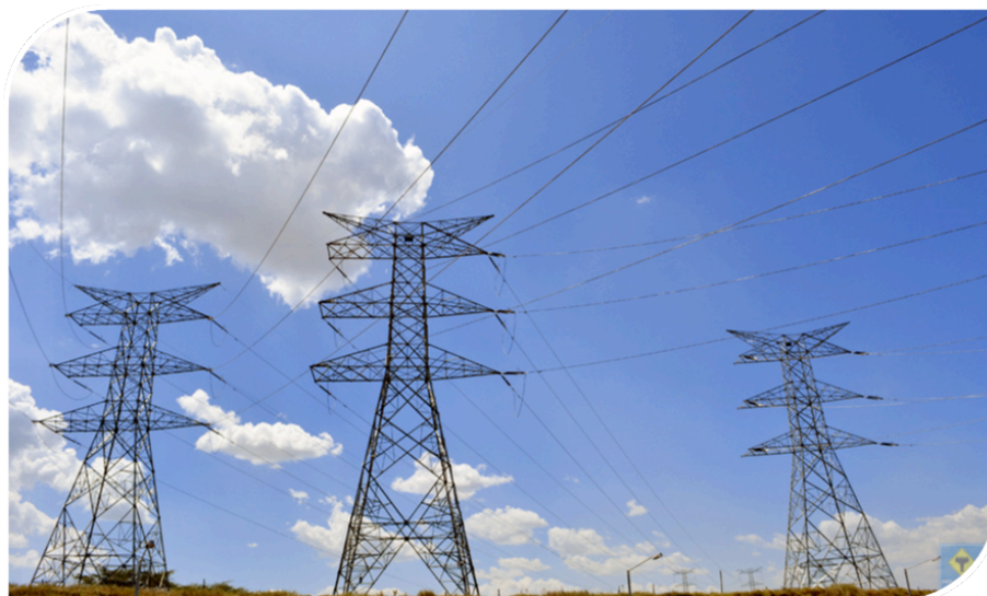
Figure 17: High Voltage Transmission Power Lines
