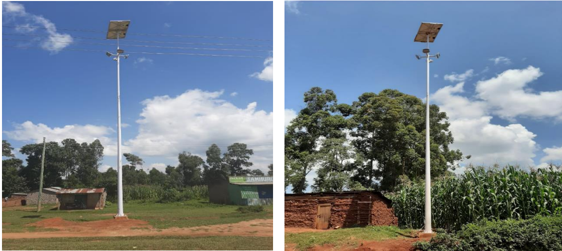
Plate 7: Streetlights installed along markets and highways to enhance on security and promote 24hr economic.
