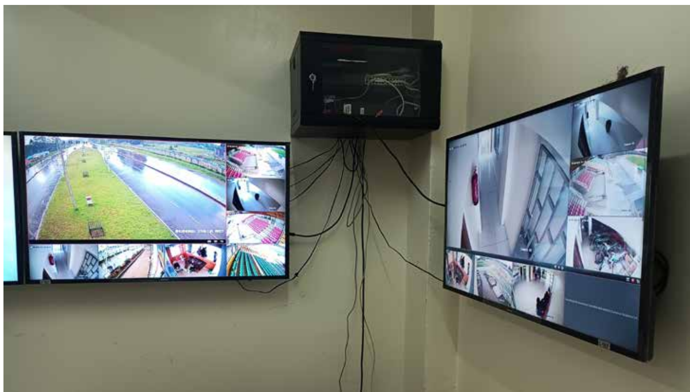
Photo 15: Central security surveillance systems control centre
