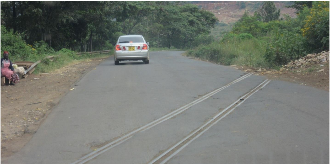
Figure 55: Abandoned railway line crossing the C71 south of Murang'a
