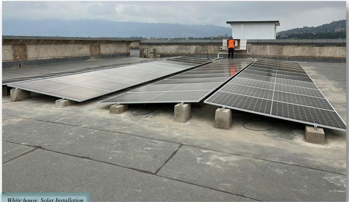
White house, Solar Installation
