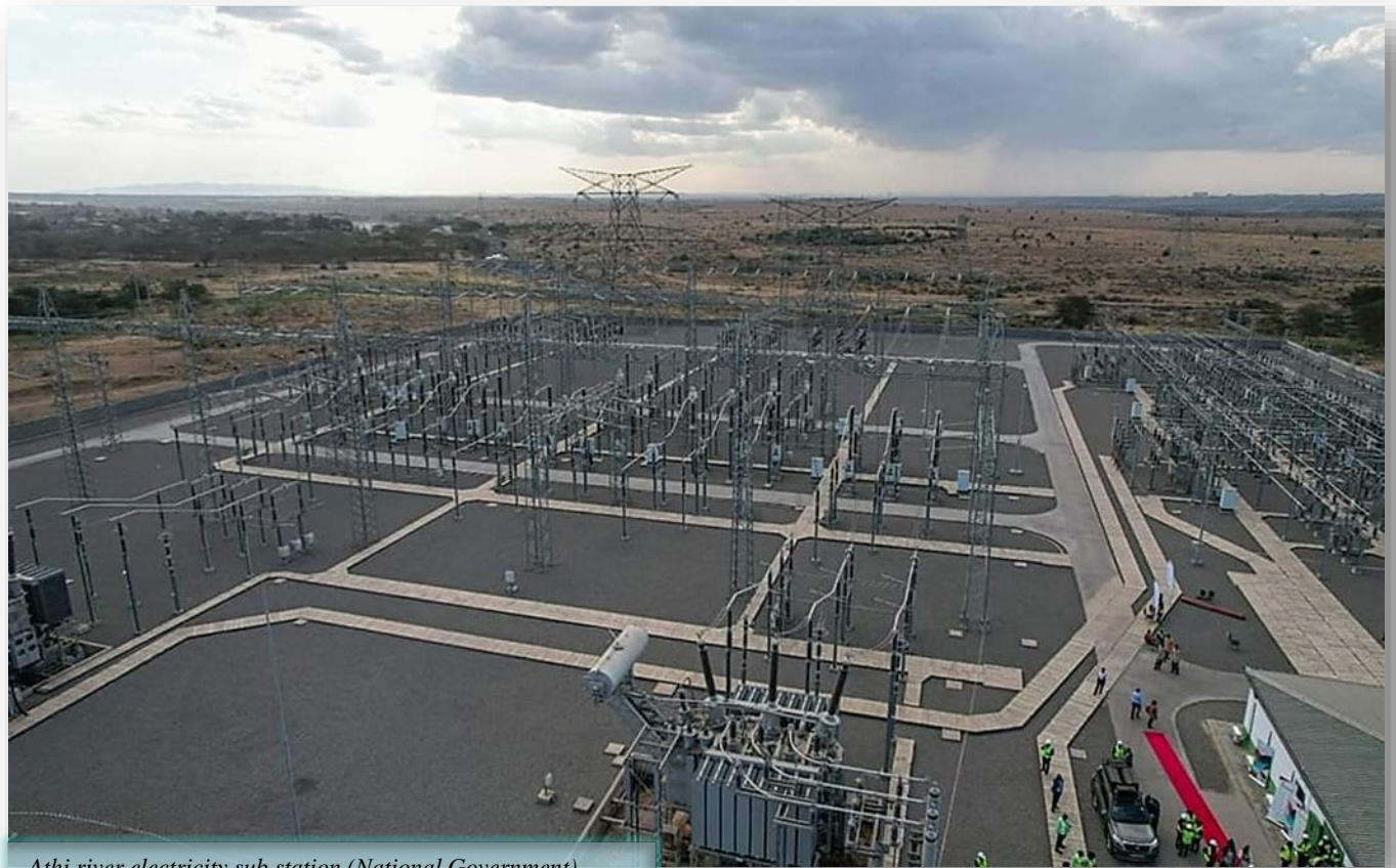
Athi river electricity sub station (National Government)
