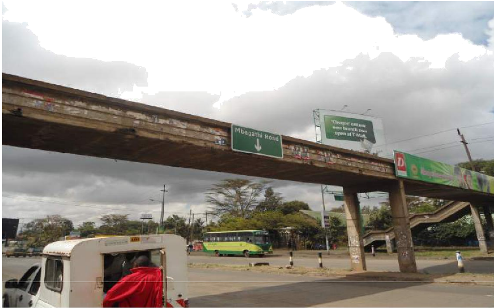
X Protrudes above the top of the road bridge: Not keeping with bridge architecture (Mbagathi footbridge)
