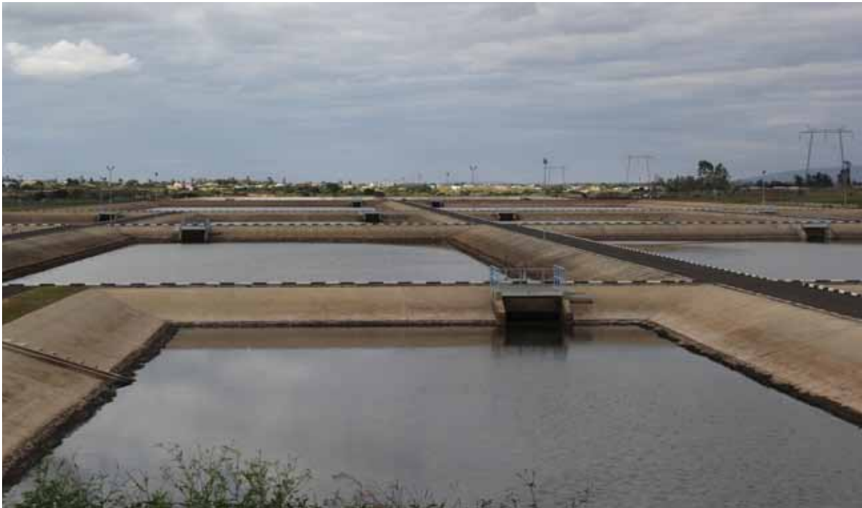
Sewerage facilities at the Ruiru-Juja Water and Sewerage Company
