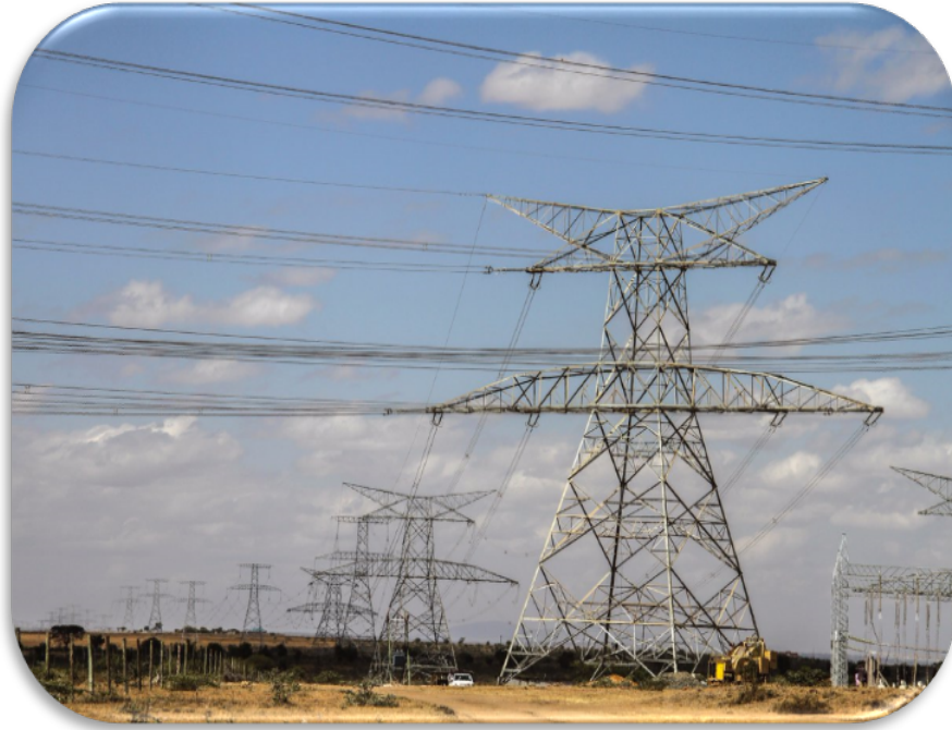
Figure 20: Newly installed high voltage power lines
