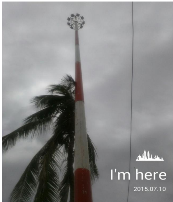
High Mast Lights
