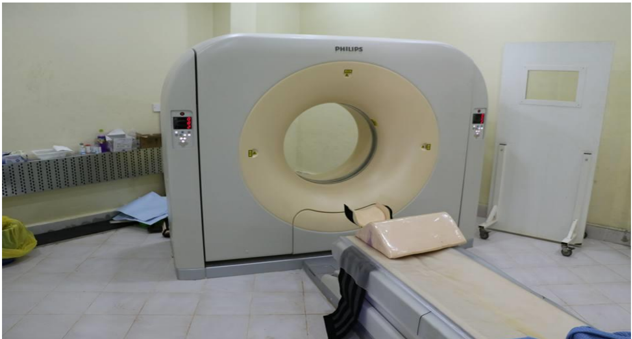
Photo 4: CT scan installed at the County General Hospital
