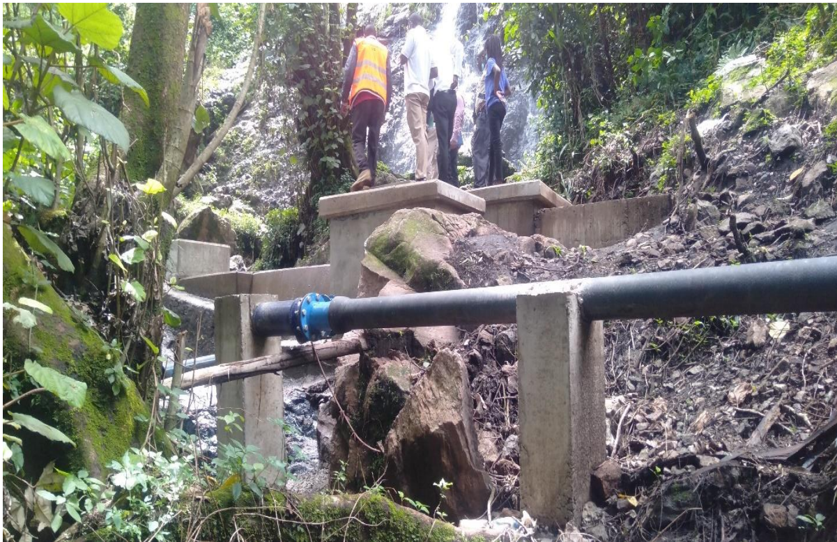
Photo 4: Augmented & Rehabilitated 6M wide intake Weir and Raw water mains and Gravity Raw Water (160M long) 180MM diameter at Kuvasali Water Project-100% done
