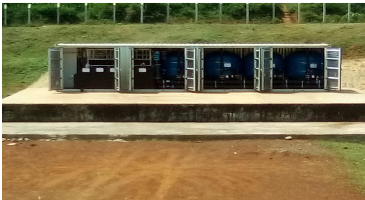
Photo 5: A containerized treatment plant Musembe Dam Water Supply Project
