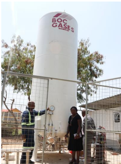
Plate 15: Gas Plant at JOOTRH
