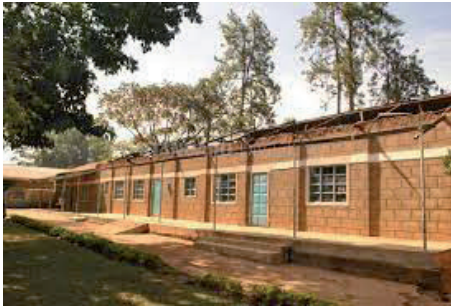
(a) Mary's St Shibuye Girls Primary Schools roof of classrooms blown off by wind (Photo by Duncan Ocholla/Standard)
