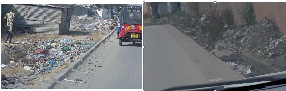
Figure 4.6: Solid waste filling storm drains
