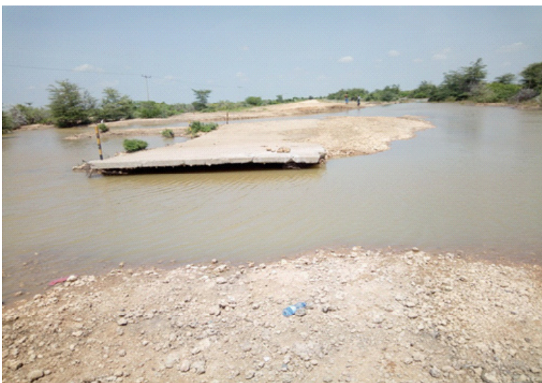
Plate 7. 4: Damaged drift connecting Habaswein-Madogashe Credits: department of disaster management and humanitarian coordination, Wajir County.
