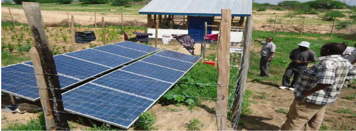
Figure 9: Solar panels in Ashabito Water Pan
