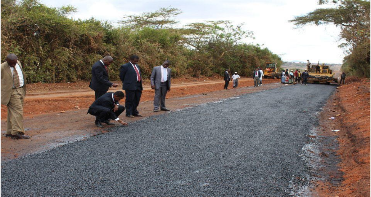
Construction of the road leading to the proposed site for the New Machakos City and Machakos Peoples Park
