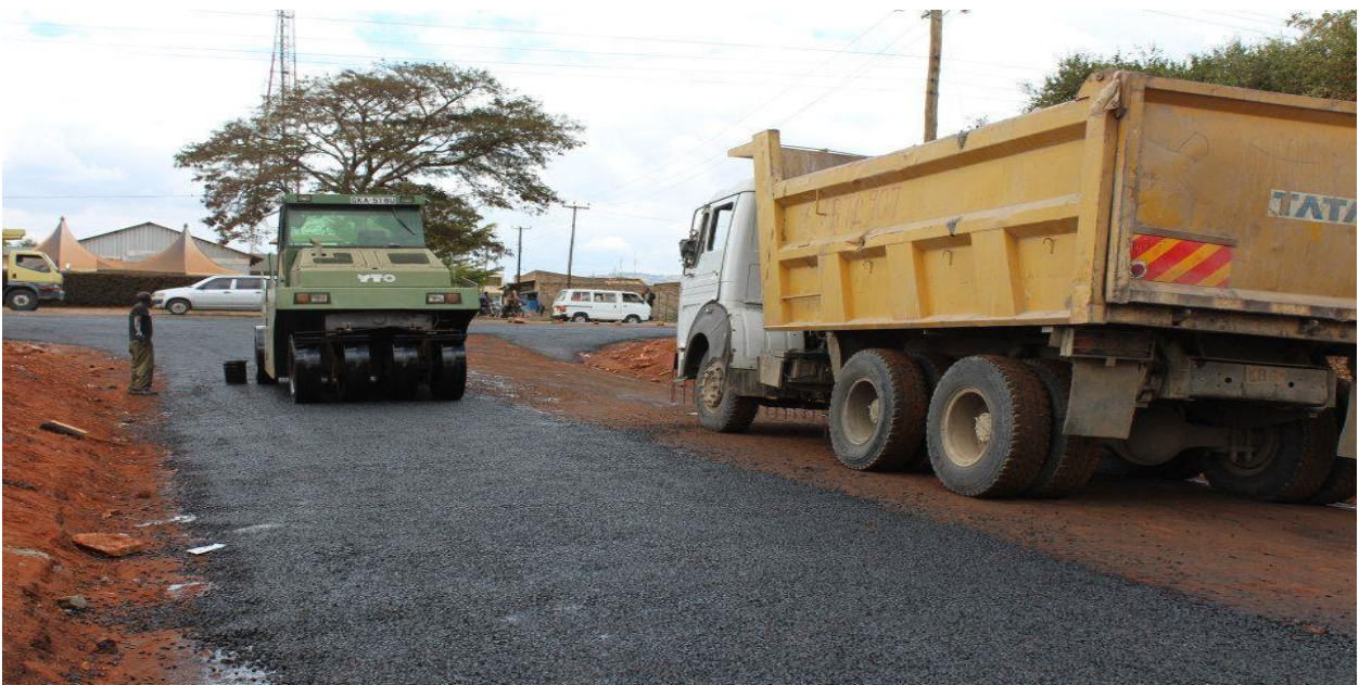
Construction of the road leading to the proposed site for the New Machakos City and Machakos Peoples Park
