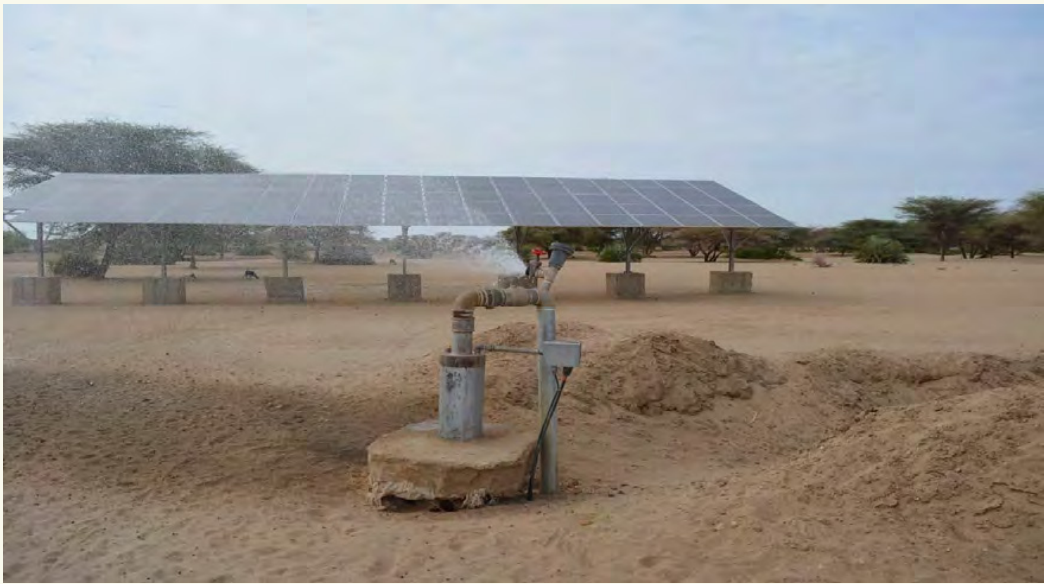
Figure 8: Solar powered water pump at the Napuu Basin within Lodwar
