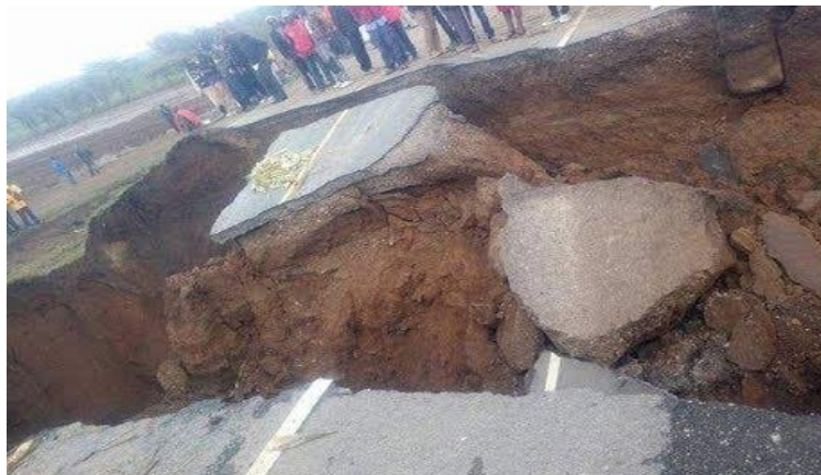
Figure 2: A section of Mai- Narok road destroyed by heavy rains
